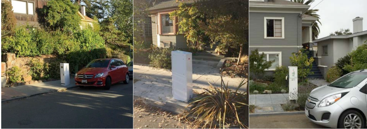
Figure 3 Examples of installed residential curbside electric vehicle charging stations. Photos courtesy of Sarah Moore, Berkeley Residential Curbside EV Charging Pilot Program.
